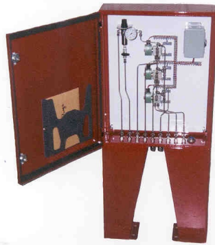
Pneumatic Solenoid Control Panel
